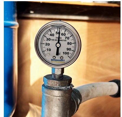
Power On Pump Check On/Off Settings
